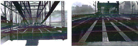
Replacing the roadbed and deck on the downstream side of the Smithfield Street Bridge in 1933. fig. 2 Smithfield Street Bridge renovation, 1933. Photo online from Brookline Connection. 4
