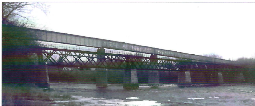
fig. 6 Massena rail bridges crossing the Grasse River, truss bridge in foreground, girder bridge in background. Photo credit Russ Nelson. 9
